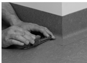
Cut out the floor covering that will be laid on top of the skirting
